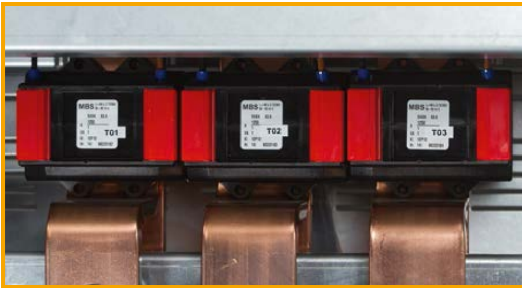
Fig. 9 Protection current transformer set
