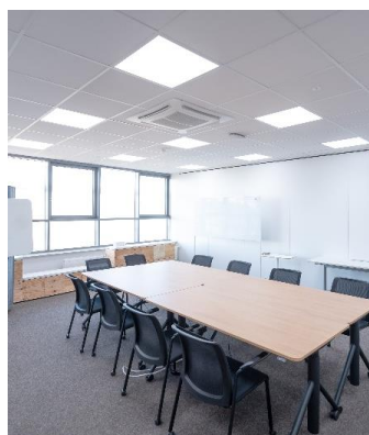
Meeting room with DALI light and sensor control
