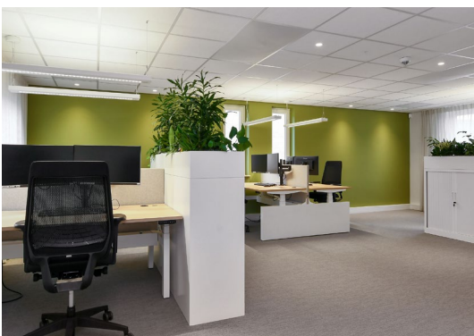
High-precision lighting for concentrated work: UGR \leq 19 downlights with beam angles from 55^\circ to 60^\circ provide glare-free lighting in modern working environments.
